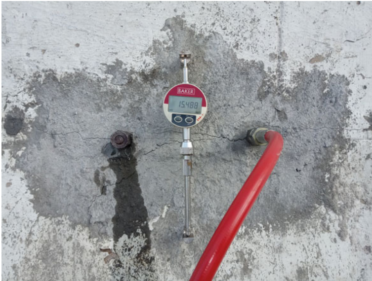
Photo 3 Placing of dial gauge after fixing flat jack between the two pins
