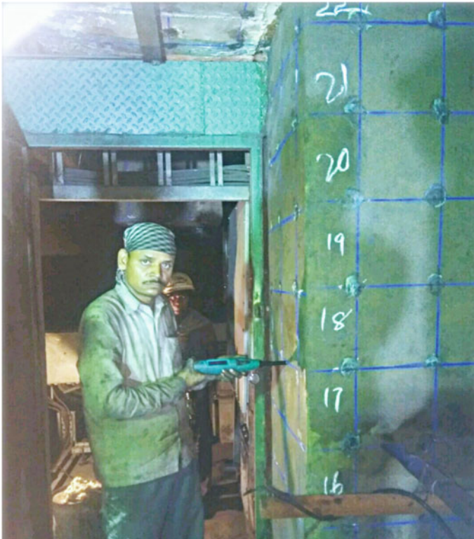
Fig. 6 In-situ rebound hammer test for cone column is in progress at site
