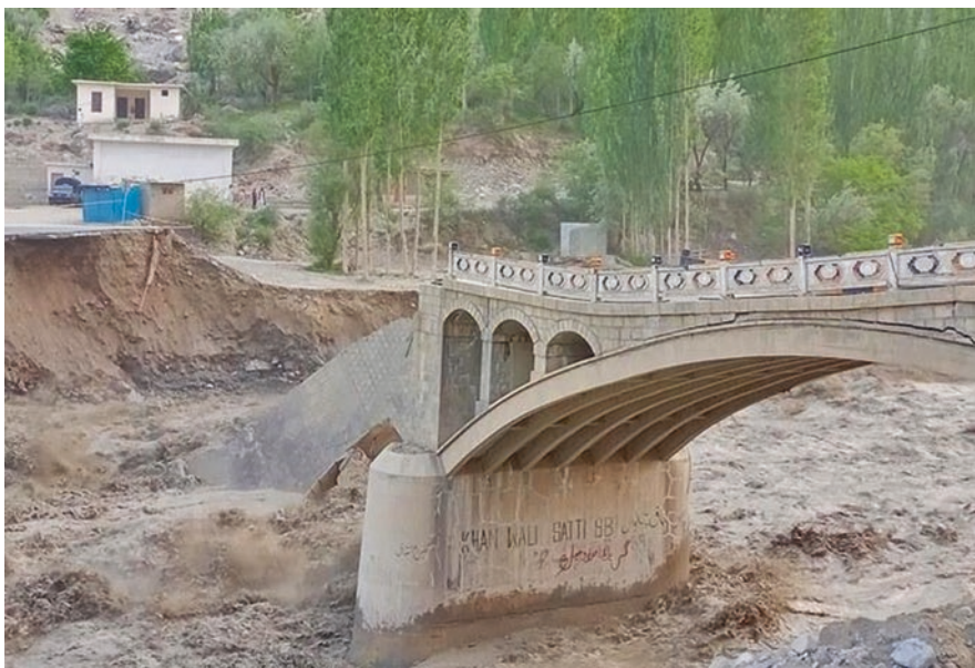
Fig. 9 Infrastructure damage due to flooding
