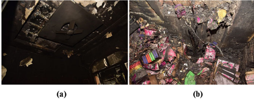
Fig. 22.3 (a) Presence of smoke and (b) destruction caused by fire
