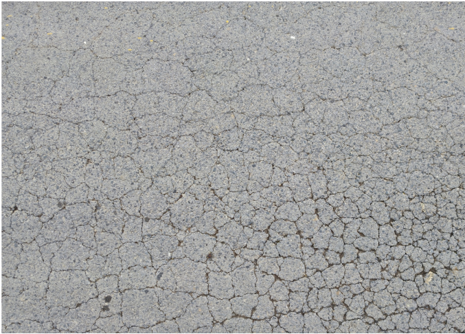
Fig. 7.21 Fatigue cracking in asphalt pavements
