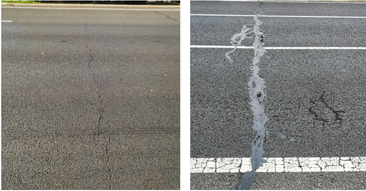
Fig. 7.19 Thermal cracking on asphalt pavements
