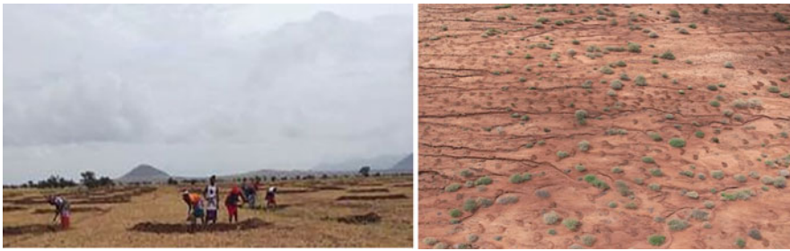
Fig. 3.14 Restoration activities in Mbirikani: bunds construction in Ilchalai (L), constructed bunds in Loosikitok (R) (Photos: BLF 2021)
