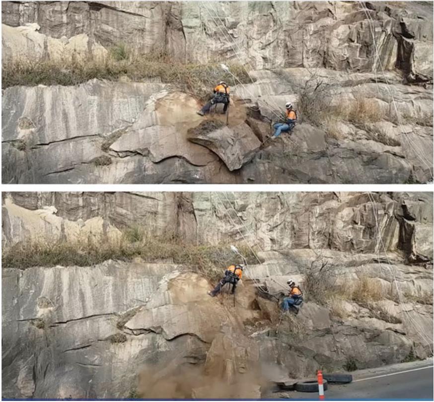
Fig. 7 Removal process of a potentially unstable rock block (after TfNSW website)
