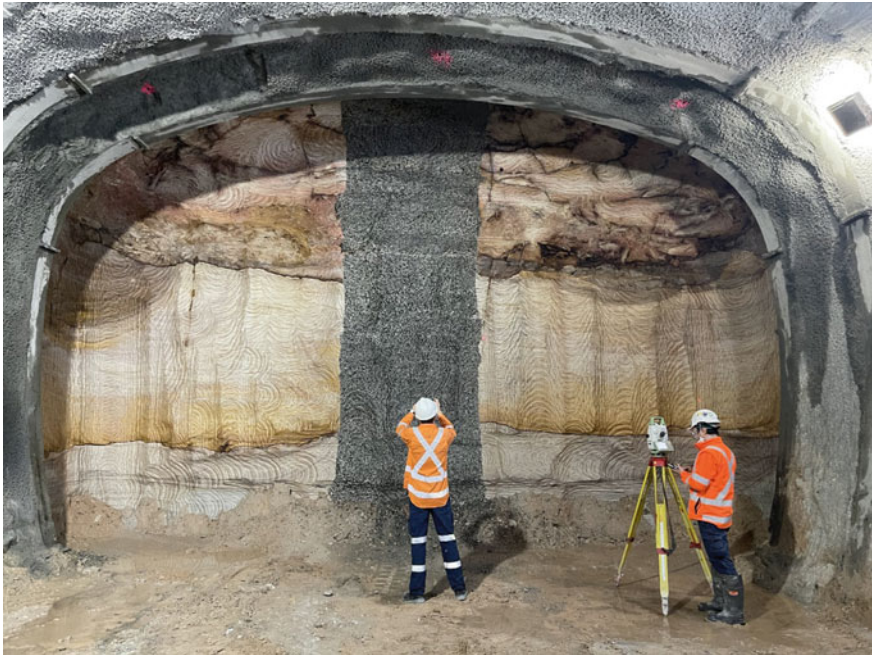
Fig. 12 Initial advance below C10 showing MCB extending below tunnel invert
