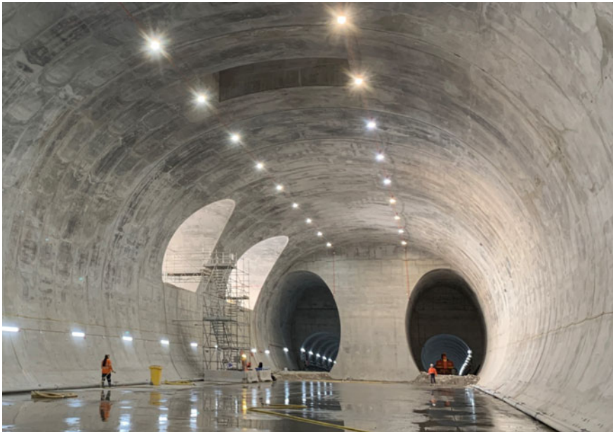
Fig. 9 Completed permanent lining with lift shaft opening evident in the crown (9 November 2020)
