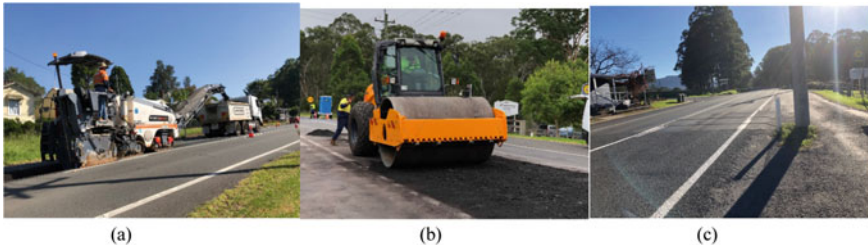
Fig. 27 Construction sequences a Removal of existing layer, b compaction using Roller, c complete surface
