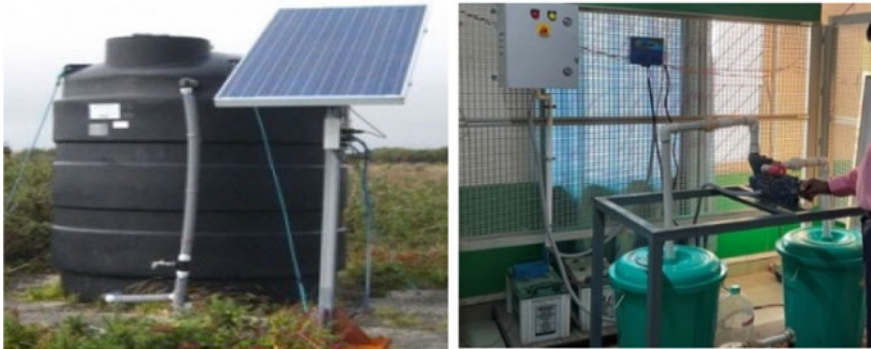
Fig. 6 0.5 HP and 1 HP solar water pumping system at CUTM, Odisha
