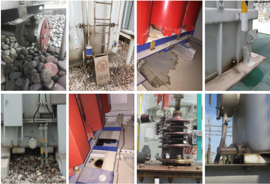
Fig. 1. Schematic diagram of oil leakage from substation equipment. In the picture, the background of the oil leakage part is complicated and the color is darker
