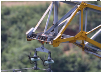
(c) Missing pins
