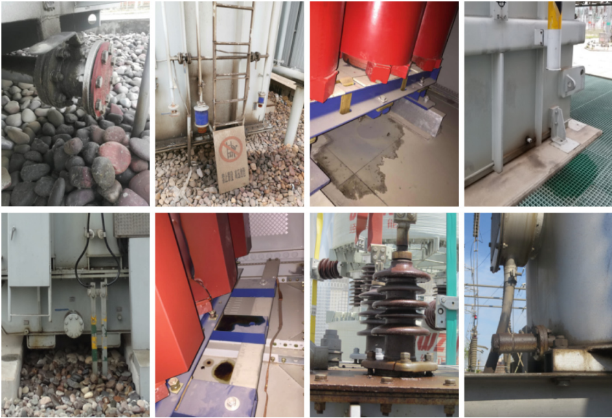
Fig. 1. Schematic diagram of oil leakage from substation equipment. In the picture, the background of the oil leakage part is complicated and the color is darker
