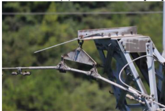
(b) Missing nuts
