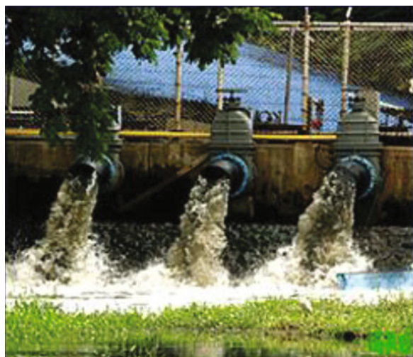
Fig. 17.1 Wastewater from industries is released directly in water bodies
