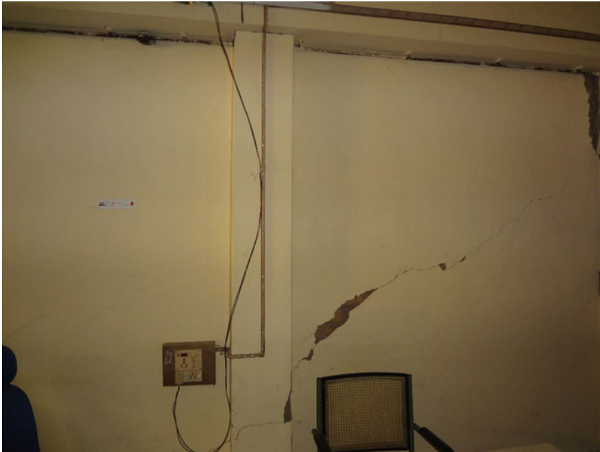
Fig. 13.1 Diagonal cracking in an infill panel and shear failure in adjacent column
