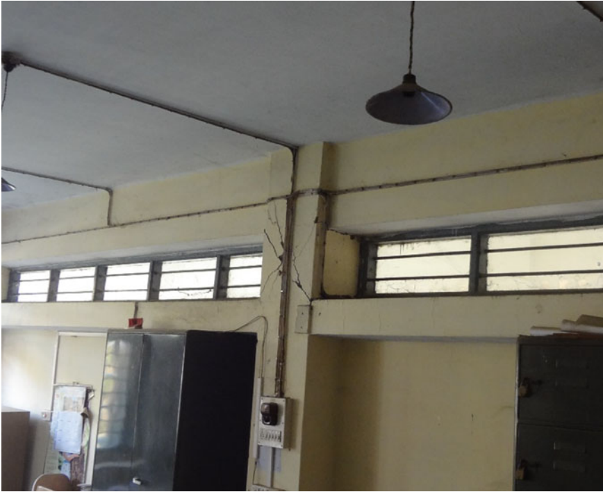
Fig. 13.2 Shear failure of columns due to partial infills
