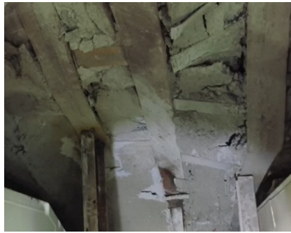
Fig. 2. Soft rock tunnel deformation causing distortion of steel arch frames.
