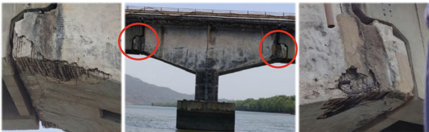
Fig. 19 Hammerhead portion, showing corrosion damages at the end articulations
