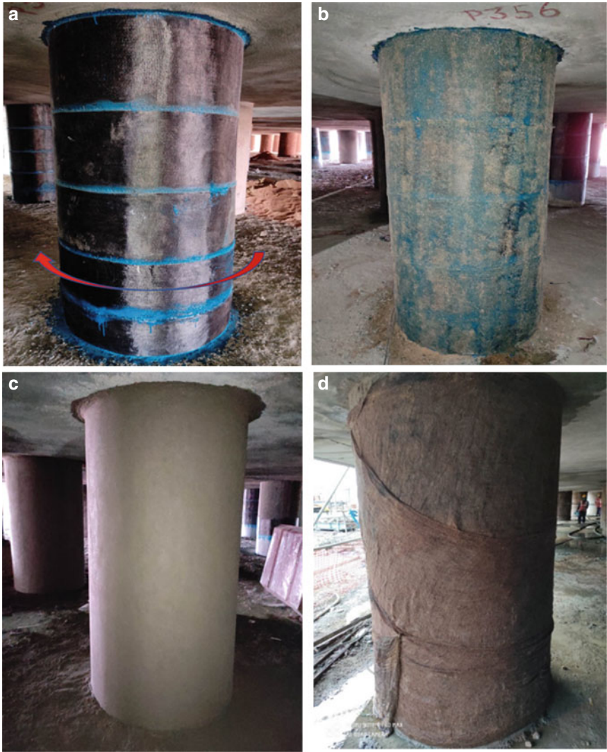
Fig. 18 a FRP Wrapping for confinement, b Sand pasting for adhesion, c Cementitious protective plastering d Curing using wet gunny bags for protective plastering
