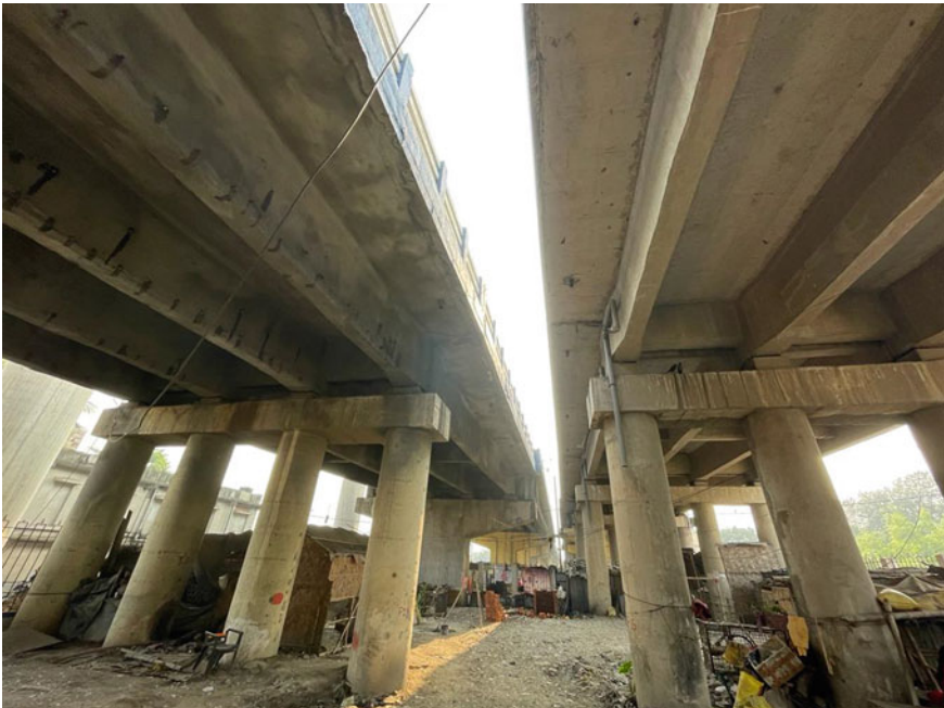
Fig. 5 A portion of Baghajatin flyover showing the old and new bridges side by side
