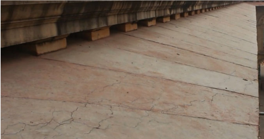
Fig. 27 The lime concrete chajja of Rashtrapati bhavan showing distresses due to corrosion
