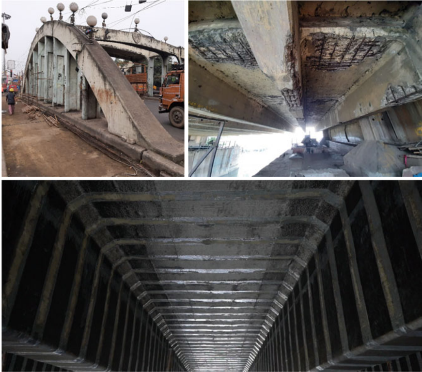
Fig. 1 Before and after structural repairs and FRP based retrofitting measures were performed on 100-year-old Chitpore bridge in Kolkata
