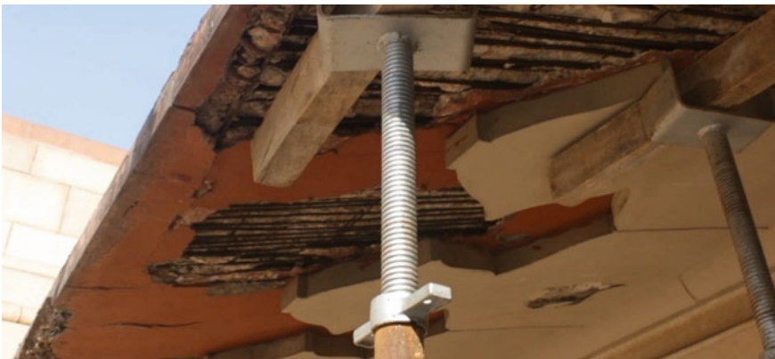
Fig. 28 Dilapidated chajjas showing spalled areas. Temporarily, external supports were given
