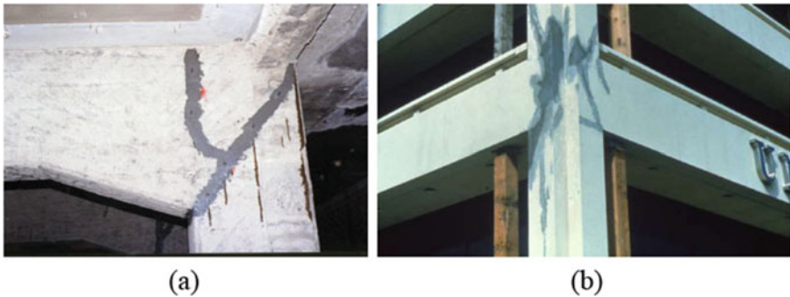
Fig. 17 Application of a epoxy resin, b cement grout injection in beam-column joints [157]
