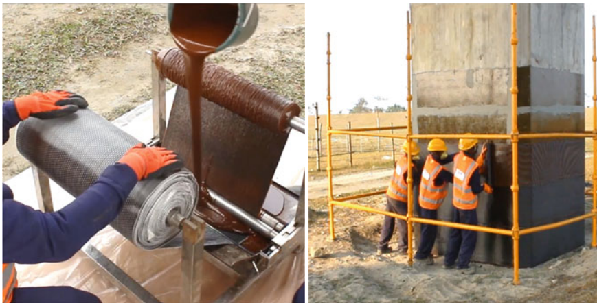
Fig. 15 Wet layup machine saturating a roll of 600 GSM unidirectional CFRP (left) and the saturated roll of CFRP being applied on the piers after application of primer (right)
