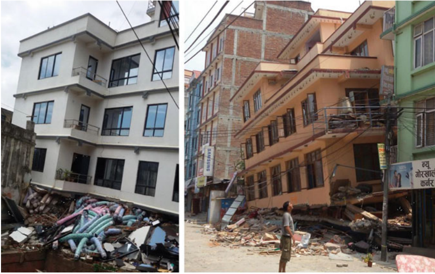
Fig. 3 Reinforced concrete buildings failure in Kathmandu, Nepal [149]
