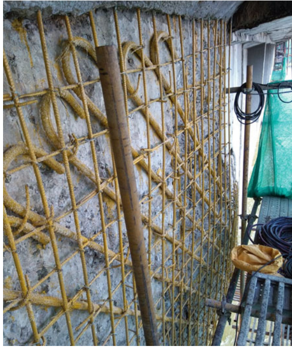
Fig. 23 Anti-corrosion treatment completed on the existing exposed steel and newly added rebars
