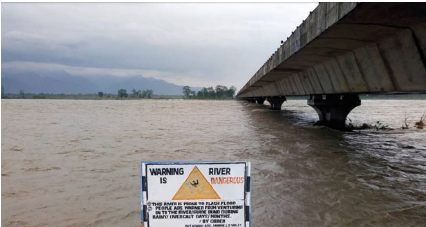
Fig. 3 Water from the melted snow and the rain, combines to reach high flood water levels, causing complete submergence of piers, exposing them to impact from floating bodies such as uprooted trees
