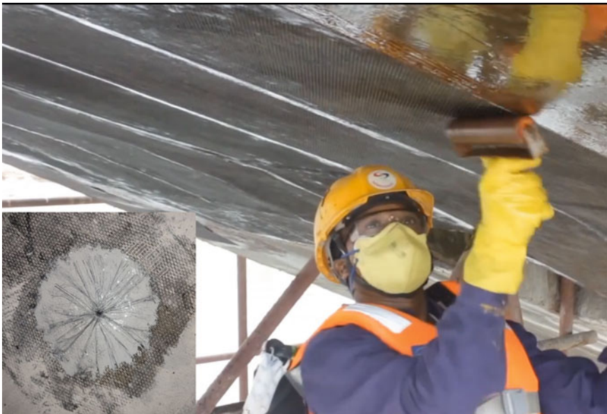
Fig. 24 CFRP being applied on the cantilevering portions of the hammerhead, Inset: Carbon anchors, installed for improving the bonding between concrete and CFRP
