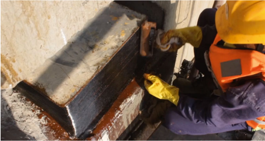
Fig. 25 Pedestal after micro-concreting, undergoing CFRP wrapping for additional confinement before installation of bearings
