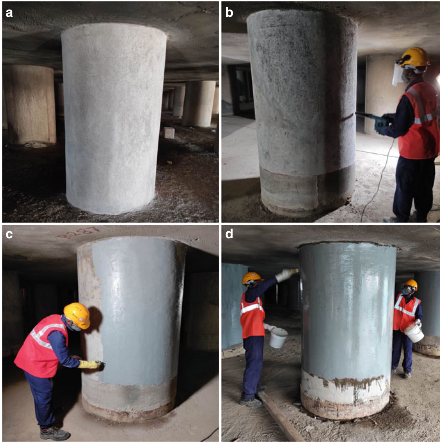
Fig. 17 Stages of surface preparation before strengthening: a Surface grinding, b Pressurized air blowing, c Structural putty application for smoothing, d Primer application
