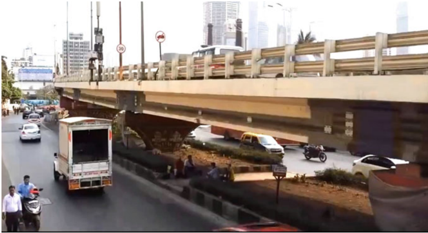
Fig. 4 Love Grove flyover in Mumbai, India showing carbon laminates exposed to direct sunlight, protected by UV resistant coating
