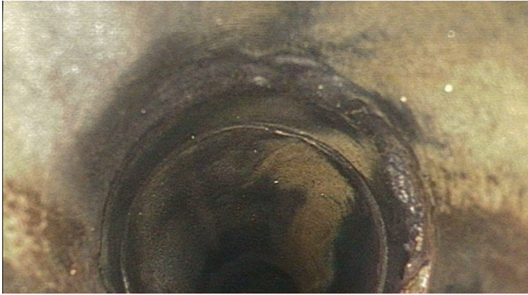
Fig. 4.3 Actual image inside boiler header for experiment 1
