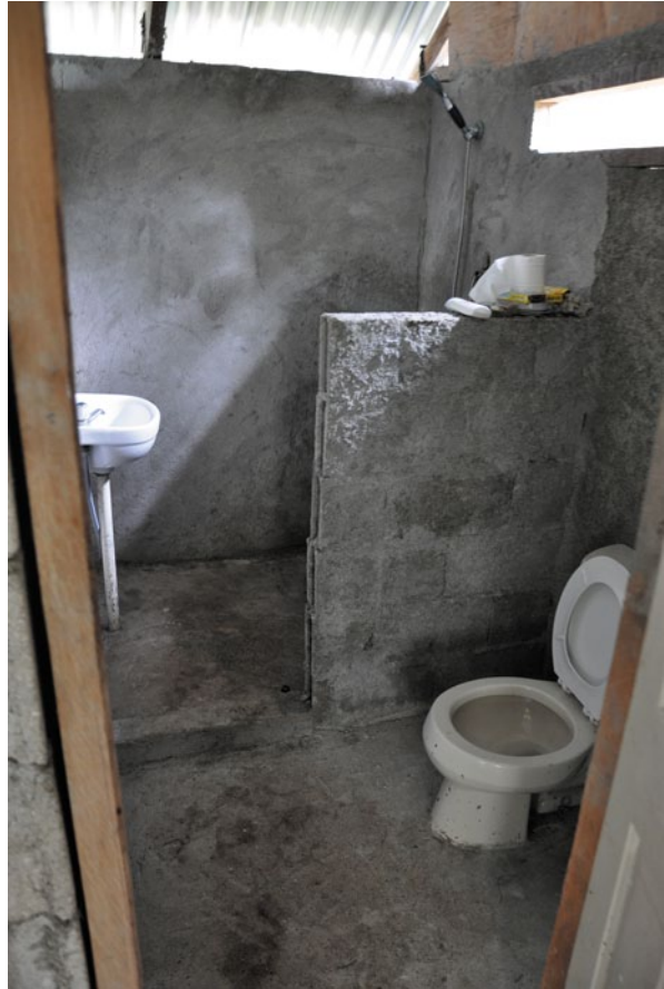
Fig. 5.12 A masonry ensuite bathroom in an existing visitor accommodation bungalow on Tanna Island provides the convenience of proximity, but has problems of overall amenity and privacy
