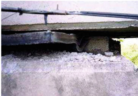
Fig. 3 The rubber bearing pad is dislocated [4]
