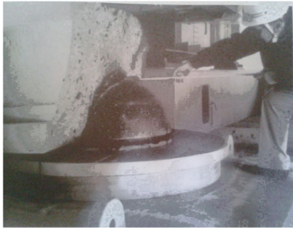
Fig. 2 Nishinomiya-ko bridge bearing failure in the 1995 HyogoKen Nanbu earthquake [5]
