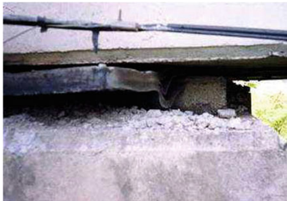
Fig. 3 The rubber bearing pad is dislocated [4]
