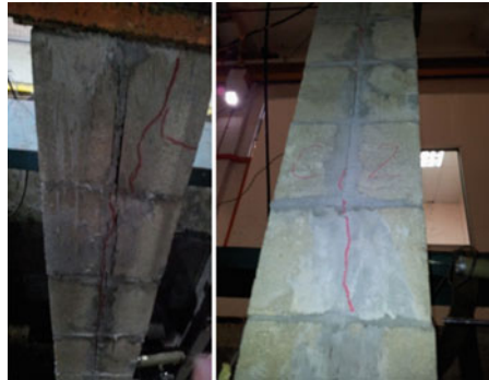
Fig. 13 Failure mode in column C2
