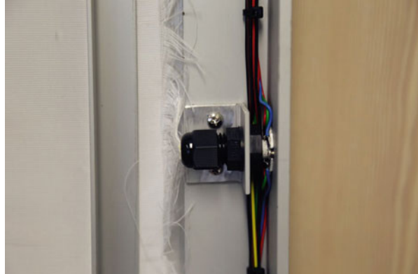
Fig. 24 Cable glands were fixed onto the frames to ensure the POFs fibers did not shift and affect the illumination
