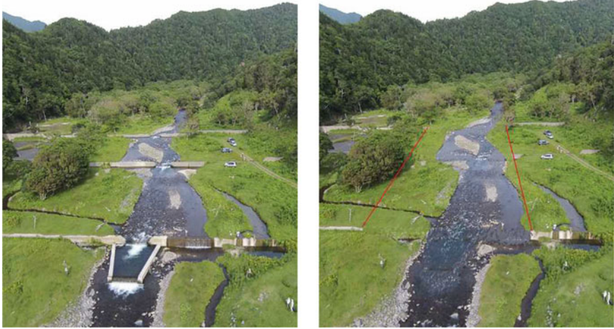
Fig. 16.6 Image of underwater concrete removal of dam at the mouth of the Rusha River (Rand 2020)
