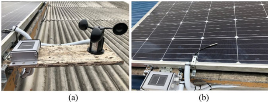
Fig. 5 Sensors installation on IoTPV system. a Irradiant and anemometer, b temperature sensor
