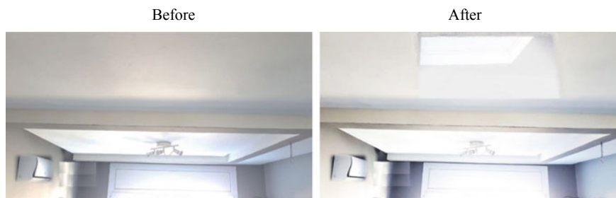
Fig. 7 North bedroom before and after opening the window. Photo of the ceiling of the studied room
