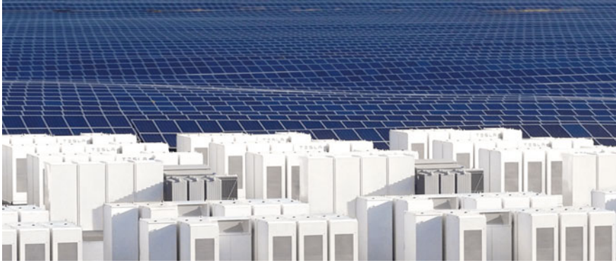
Fig. 2 Photograph of battery system for large scale solar power plant
