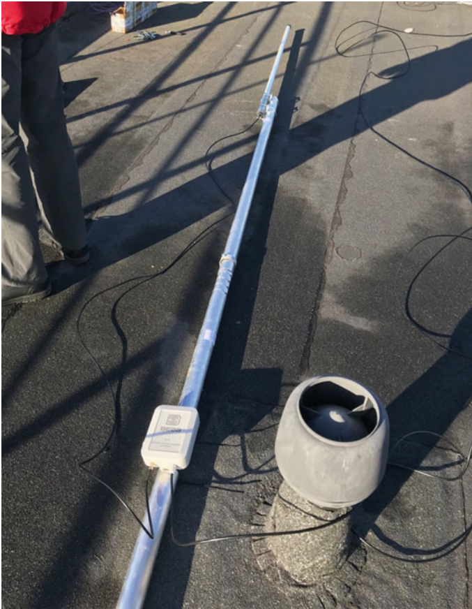
Fig. 2 LoRaWAN gateway and antenna
