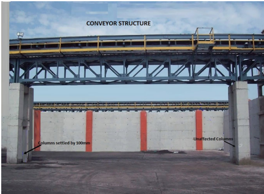
Fig. 1 Settled columns supporting conveyor structure
