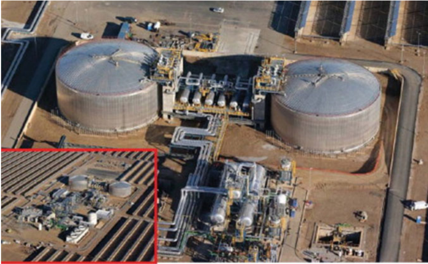
Fig. 9.8 Two-tank molten salt storage of Andasol solar power station located in Spain [16]
