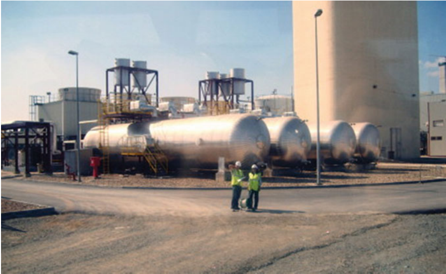
Fig. 9.10 Steam accumulators of PS10 power tower plant, Spain [16]
