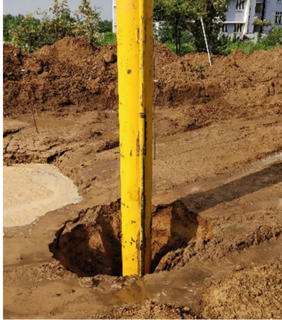
Fig. 7 Depth vibrator in action and subsidence in the form of conical carter due to compaction
