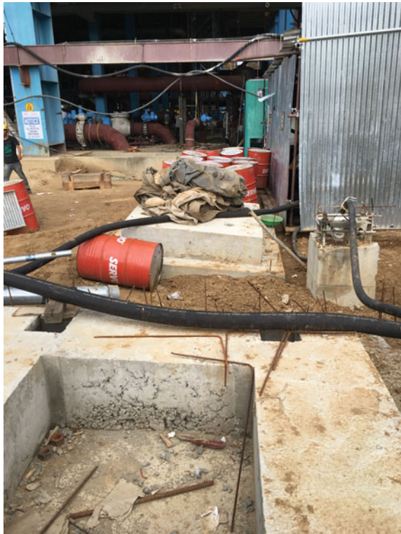
Fig. 2 Tilted foundation due to settlement
