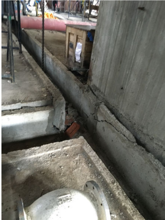
Fig. 1 Cracks in the seal oil foundation
