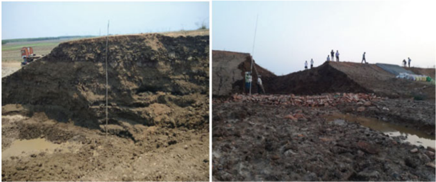
Fig. 2 Photographs showing breached sections of summer storage (SS) tank
