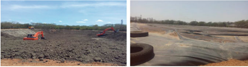
Fig. 1 Preparation of slope for leachate pond and placing of geomembrane at slope
