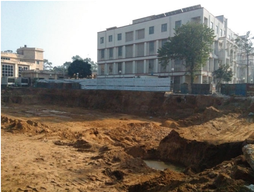
Fig. 1 Unsupported excavation adjacent to an existing building
