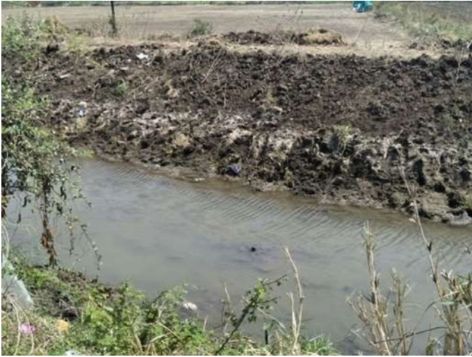
Fig. 1 Canal slope failure
