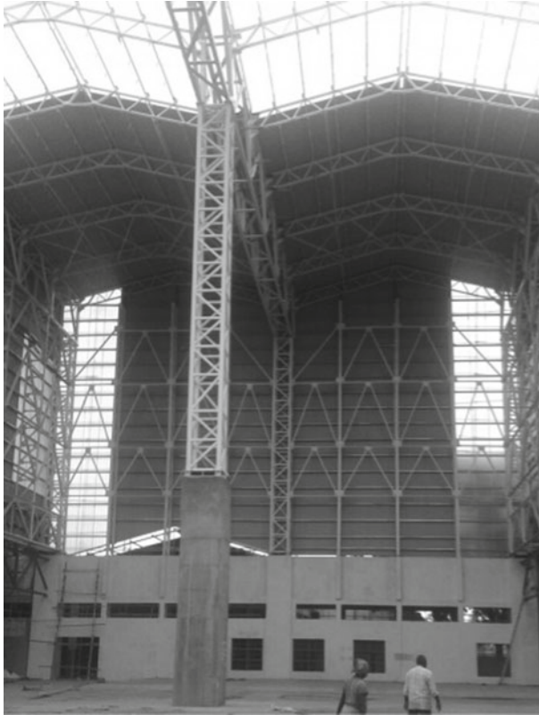
Fig. 7 Site photographs showing the erected steel structure on renovated RC column over the Underpinned foundation
