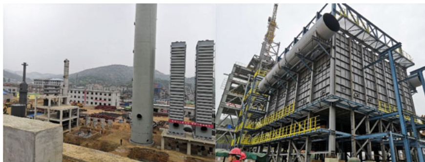
Fig. 7.14 Demo project of coke oven gas DRI co-built by China university of petroleum, sinopec and China Shanxi Taihang mining in Zuoquan, Shanxi. Source Zhou Hongjun, China university of petroleum
