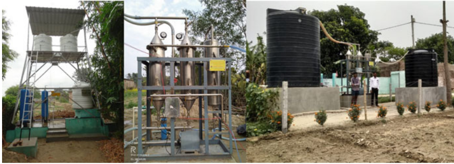
Fig. 7.20 Arsenic filters installed in Buxar and Saran districts of Bihar
