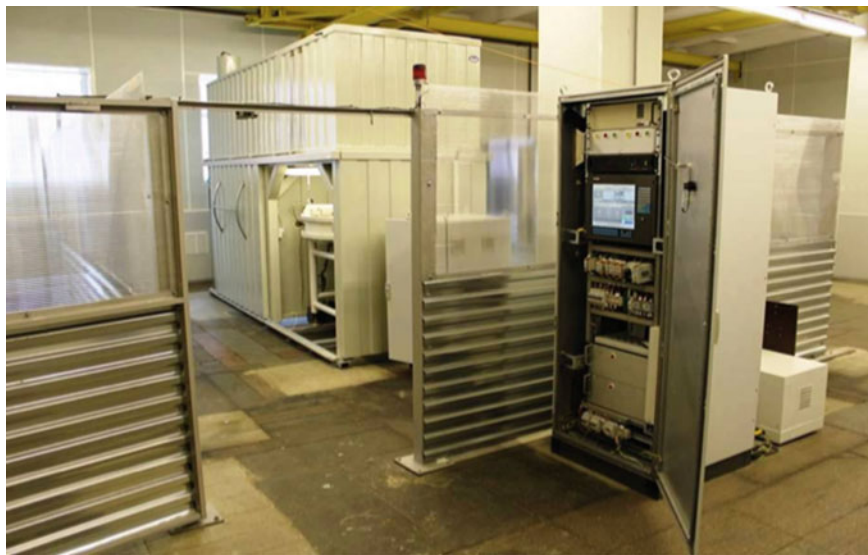
Fig. 1 Appearance of the “GEZA-MMP” installation
