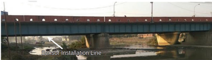
Fig. 5 Sensor installation site
