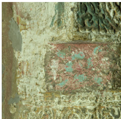
(b) Detail on the rear of the right column showing red and green paint
