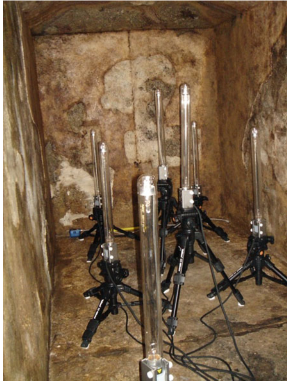
Fig. 16.9 Use of germicidal lamps in the Kitora tumulus in 2004 after removal of the plaster
