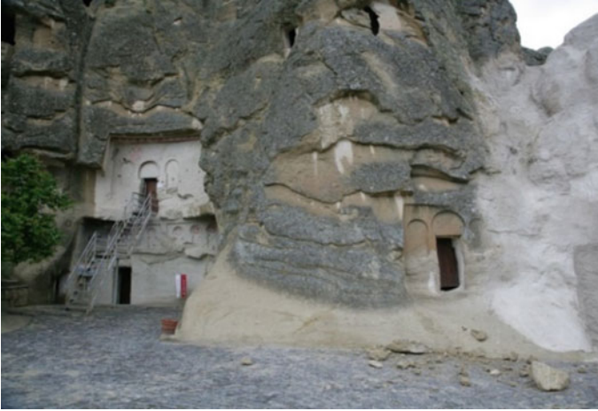
Fig. 3.8 a Çarıklı Church, Göreme Open Air Museum. Climatic factors such as wind, rain and frost cause fracturing and cracking of the surface of the tuff rocks. b Çarıklı Church, Göreme Open Air Museum. Loose rock is a potential danger for visitors
