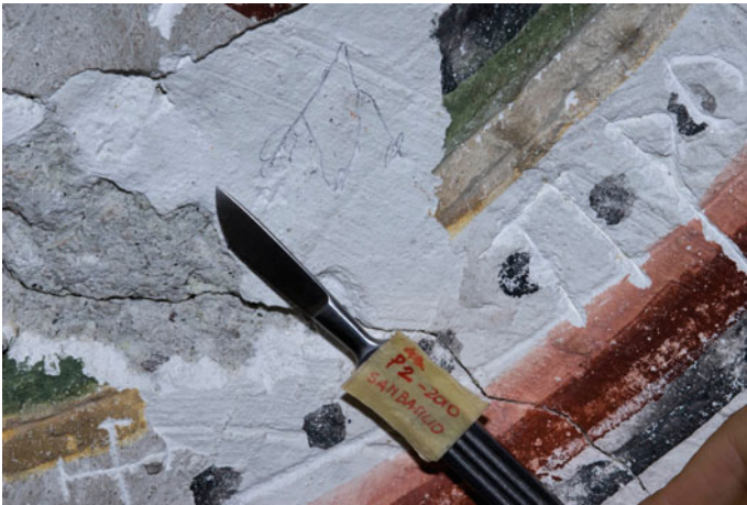
Fig. 4.23 Gomed valley, church of San Basil. Detail of the apse painting showing the overlap of the preparatory layers
