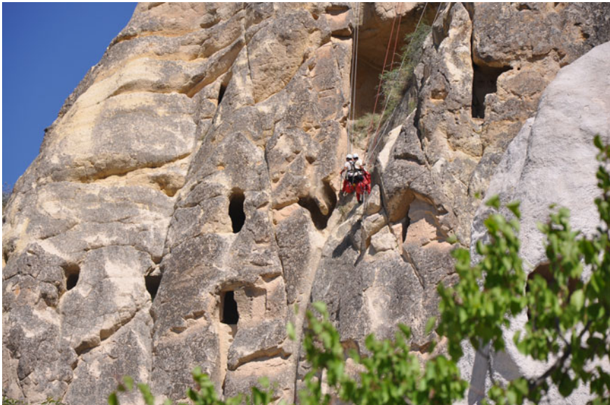
Fig. 3.10 Hidden cracks and loose rocks around the Çarıklı Church complex were completely cleaned by expert mountaineers
