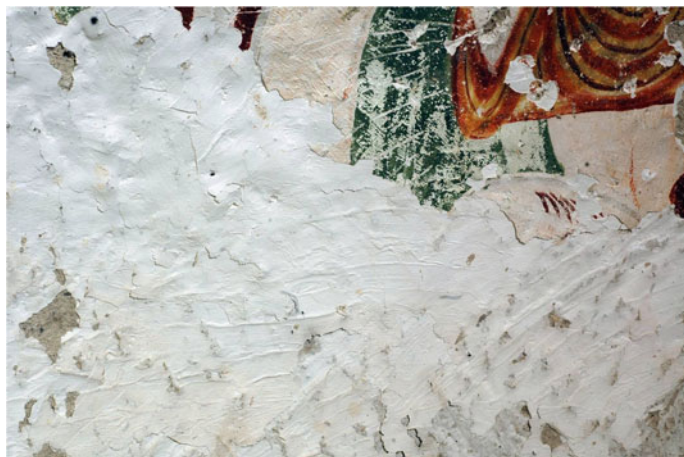
Fig. 4.25 Kızılcukur valley, church of Saints Joachim and Anna. Detail of the apse painting showing the overlap of the preparatory layers
