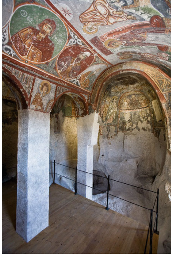
Fig. 4.7 Şahinefendi, church of the Forty Martyrs. View of the south aisle and south apse after restoration
