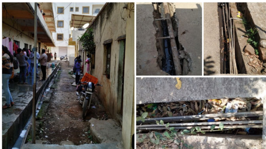
Fig. 6 Photographs showing conflicts among four systems in the Vadgaon Maval
