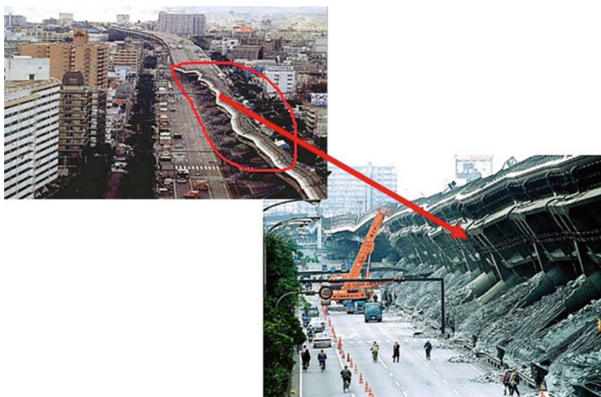
Fig. 3 Hanshin Expressway collapse during Kobe Earthquake, 1995 [30]
