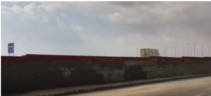
Fig. 1 Reinforced earth wall in saturated backfill after rainfall
