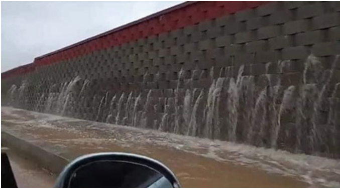
Fig. 2 Outflow of drained water through RE wall
