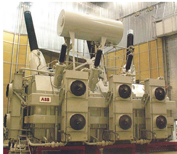
Fig. 7.85 220/110/10 kV and 250 MVA autotransformer [7.38]
