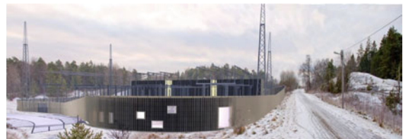
Fig. 11.23 Anneberg 400/220 kV Substation, Swedish National Grid (Courtesy Tennet/Movares)
