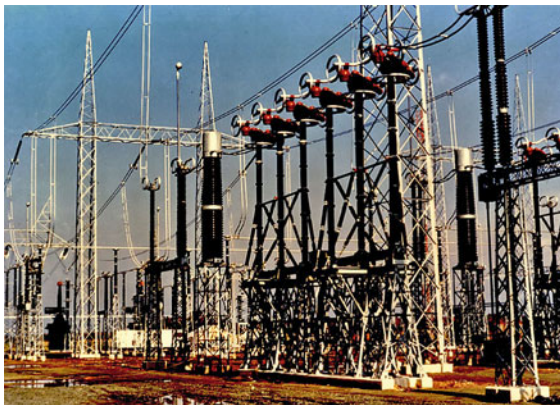
Fig. 8.34 Photograph of an example of the latest generation of 800 kV air-blast circuit breakers. (Courtesy of GE, produced by Alstom)
