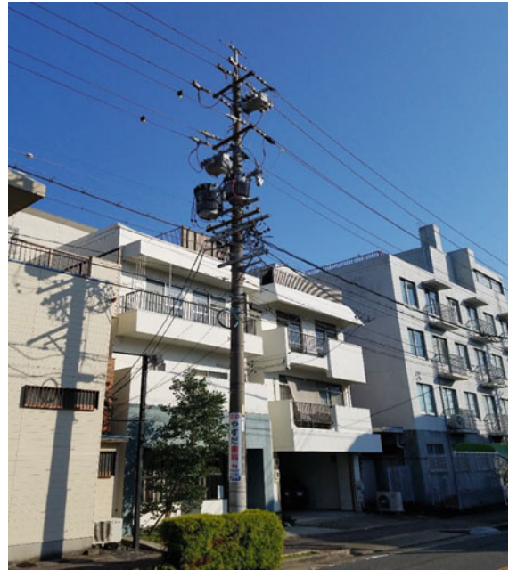
Fig. 11.7 Pole-mounted 6.6 kV substation in Nagoya, Japan, comprising switches, surge arresters, and 50 kVA and 75 kVA transformers (Courtesy Chubu Electric)
