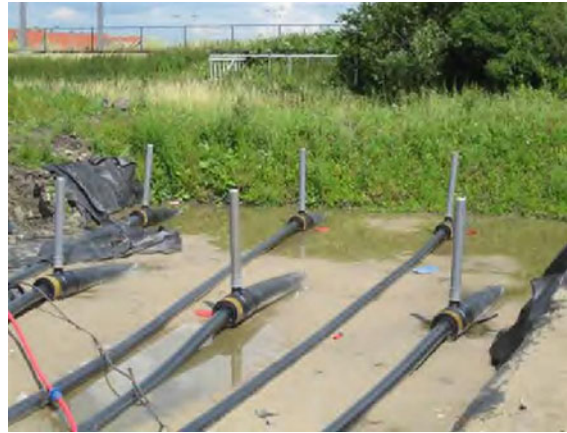
Fig. 10.100 HDD for a 380 kV cable circuit with six individual drillings (adapted from [10.14])
