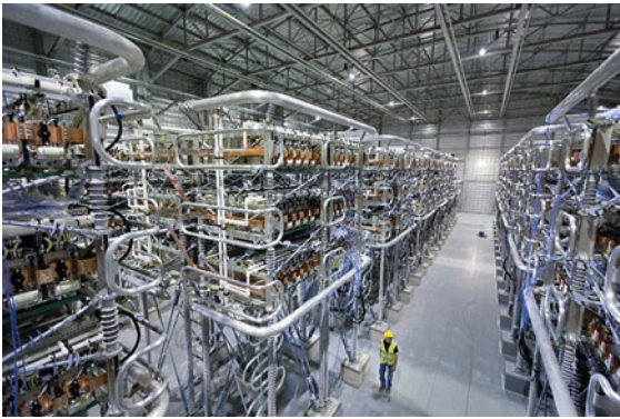
Fig. 12.64 VSC converter (courtesy of Siemens)
