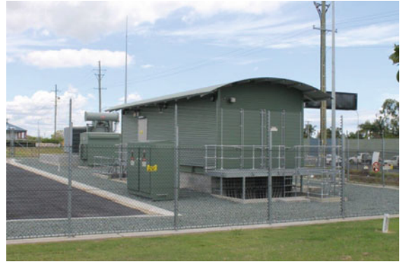
Fig. 11.42 Prefabricated substation example (Courtesy Ergon Energy, Queensland, Australia)
