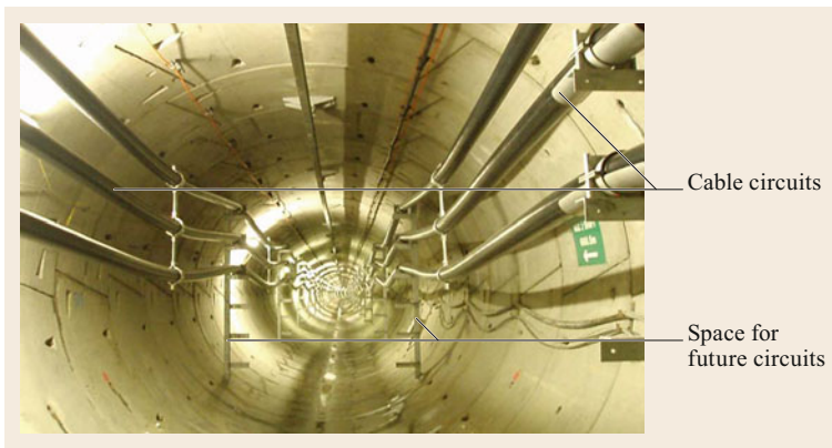
Fig. 10.12 Cables installed in a tunnel (adapted from [10.16])
