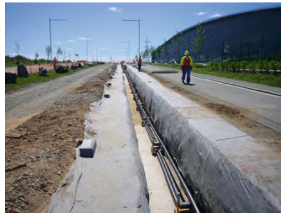
Fig. 10.90 Cables installed in an open cut trench and directly buried (adapted from [10.14])
