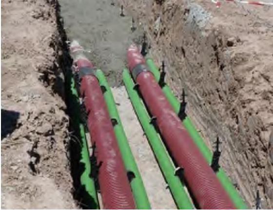
Fig. 10.93 Photograph showing the uppermost ducts (red) of two circuits (the other four ducts are under the first layer of concrete) (adapted from [10.14])
