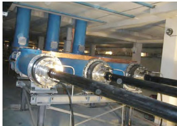
Fig. 10.88 Typical EHV GIS termination installed in a horizontal position (adapted from [10.49])
