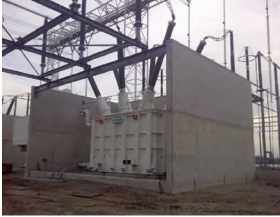
Fig. 10.49 Series reactor in a 380 kV hybrid line (adapted from [10.14])
