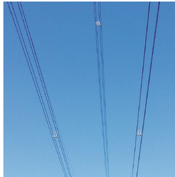
Fig. 4.68 Quad-bundled conductors with spacer dampers
