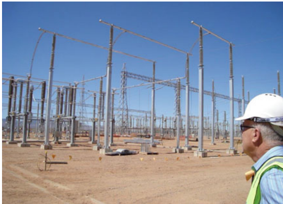
Fig. 11.19 The author inspecting a 275 kV transmission substation extension (1.5-breaker layout) under construction, Port Augusta, South Australia (Courtesy Peter Burnell)
