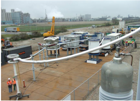
Fig. 10.113 On-site commissioning test performed with three mobile test sets simultaneously due to the cable length (adapted from [10.49])
