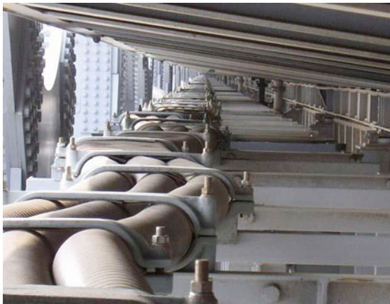
Fig. 10.14 Cables on a cable tray attached to a bridge (adapted from [10.18])
