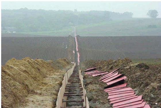
Fig. 10.9 Construction swathe for installing cables cross-country; a width of 8 m is typically required for a single trench (adapted from [10.13])
