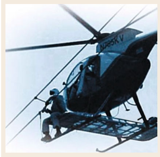
Fig. 9.172 Replacement of twin spacers on a live 500-kV line with a helicopter
