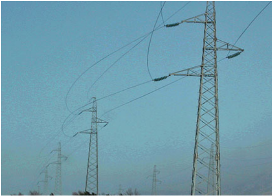
Fig. 9.15 Bora wind causes severe conductor blow-out (photo: F. Jackl)
