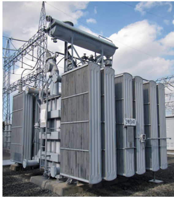
Fig. 8.22 Photograph of a 20 kV, 22.5 MVA shunt reactor bank. (Courtesy of J-POWER)
