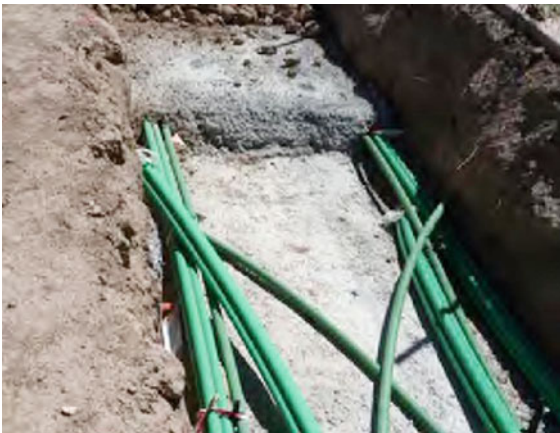
Fig. 10.94 Photograph showing communication cable ducts on top of HV circuits as well as the third (final) layer of concrete (adapted from [10.14])
