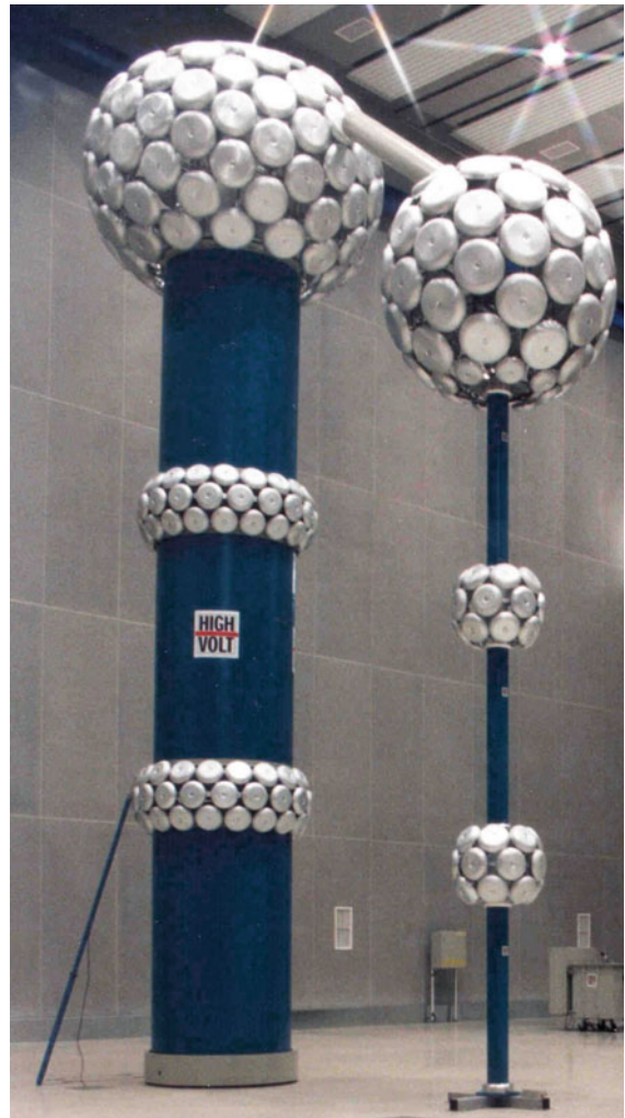
Fig. 3.42 AC transformer cascade for 1000 kV with a voltage divider (courtesy of BTU Cottbus-Senftenberg)
