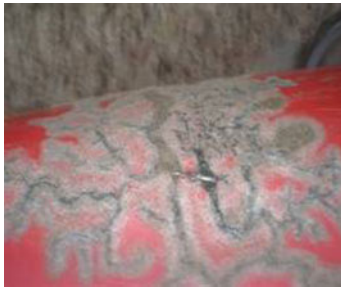
Fig. 10.114 Discharge tracks on the PE outer serving of the cable due to a defect (adapted from [10.49])
