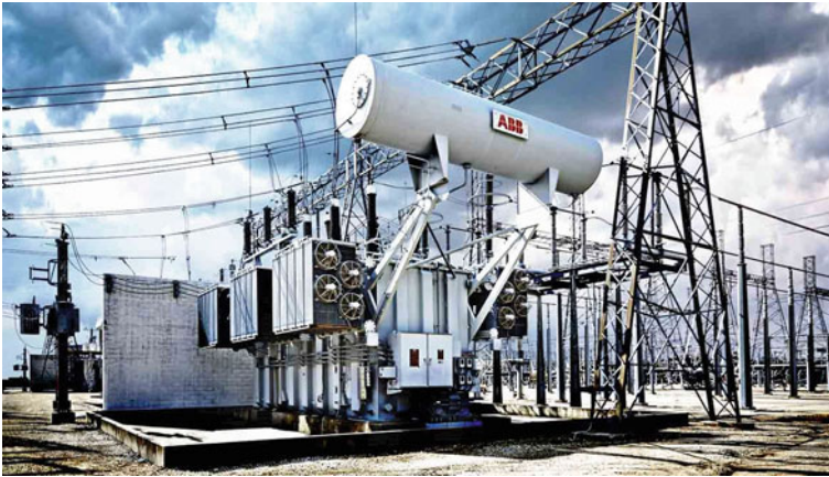
Fig. 7.83 Transformer in a substation [7.10]
