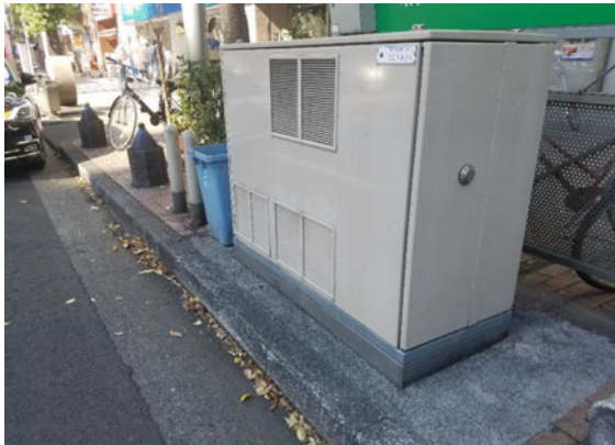
Fig. 11.6 Typical ground-level suburban 6.6 kV, 100 kV distribution substation in Nagoya, Japan (Courtesy Chubu Electric)
