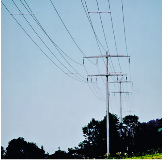
Fig. 9.101 IPSs enable the addition of a second 12-kV circuit on an existing 50/12-kV line in Switzerland
