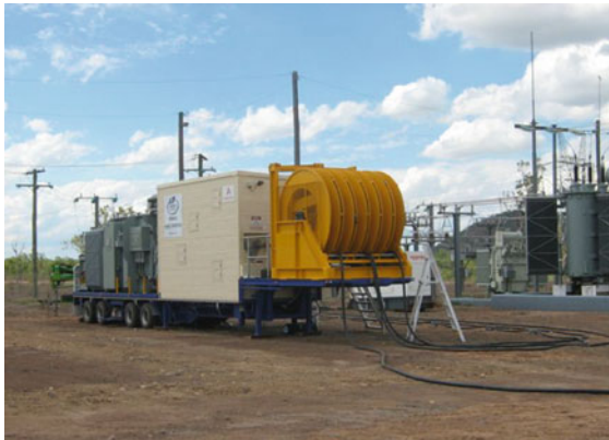
Fig. 11.39 NOMAD mobile substation in Australia in 2006 (Courtesy Ergon Energy, Australia)
