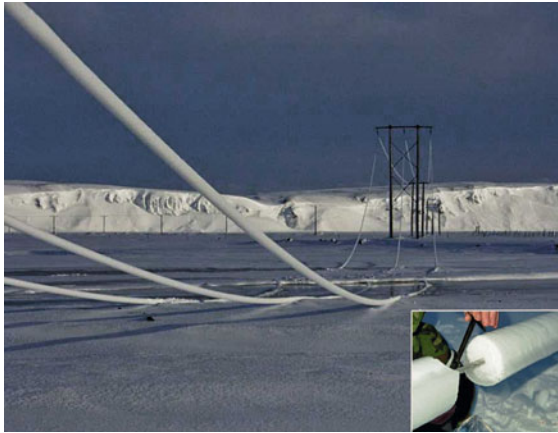
Fig. 9.13 Extreme ice accretion on line conductors leading to line outage (photo: Landsnet, Iceland)
