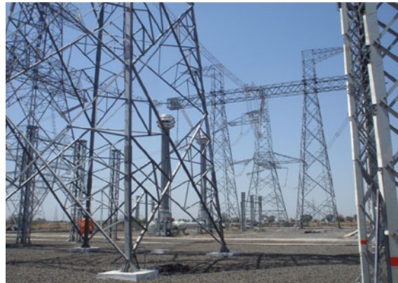
Fig. 11.4 1200 kV Bina National Test Substation, Madhya Pradesh, India (Photo: Krieg)
