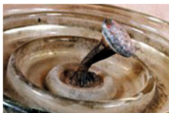
Fig. 9.74 Corroded pin of a glass cap-and-pin insulator; note the reduced diameter of the pin and the rust products at the boundary with the dielectric
