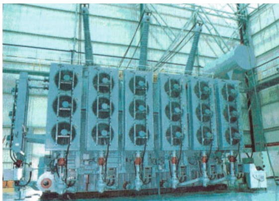
Fig. 7.82 1100 MVA step-up transformer with a nominal voltage of 19 kV/345 kV [7.10]
