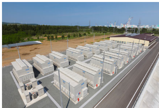
Fig. 16.39 A 34 MW Na–S storage facility in Japan (courtesy of JWD and NGK)
