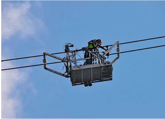
Fig. 9.168 Spacer installation on a horizontal twin bundle with the help of a cart [9.267] ◀
