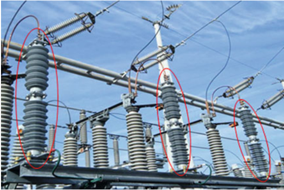
Fig. 8.7 Photograph of 77 kV composite-type MOSAs in a substation. (Courtesy of Chubu Electric Power)
