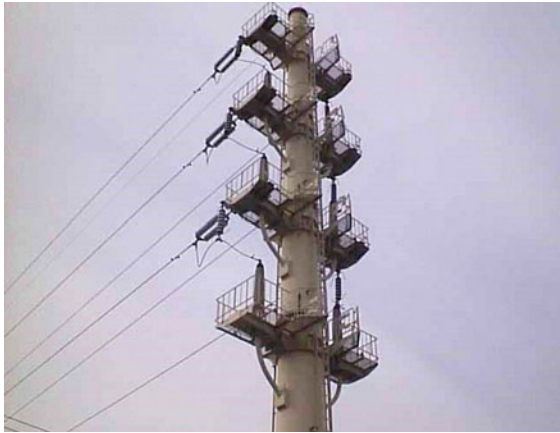
Fig. 10.7 HV terminations installed on a pole (adapted from [10.8])
