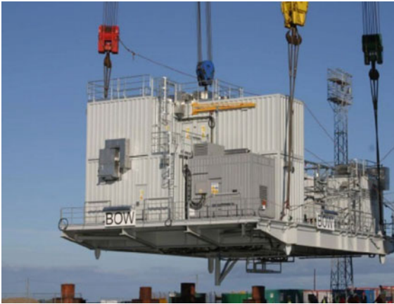
Fig. 11.40 A typical containerized substation being lifted off shore (Courtesy CIGRE [11.28])
