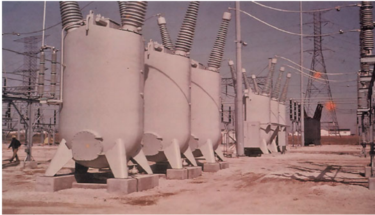
Fig. 8.33 Photograph of some 345 kV, 63 kA oil circuit breakers
