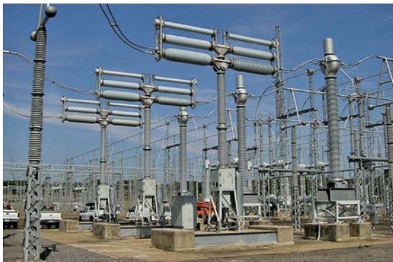
Fig. 8.4 Photograph of a 550 kV live-tank SF 6 gas circuit breaker. (Courtesy of Dominion Energy)
