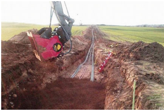
Fig. 10.8 Cables installed directly into the ground with native soil backfill (adapted from [10.15])
