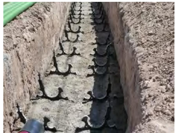
Fig. 10.92 Double-circuit trench after the first layer of concrete has been poured in (adapted from [10.14])
