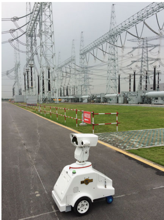
Fig. 11.44 Patrol robot in Liantang 1000 kV Substation, China (Photo: Krieg)
