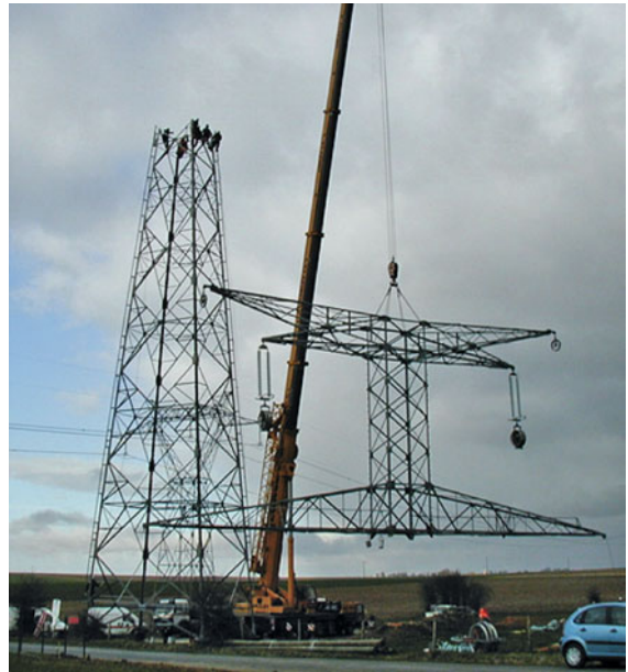
Fig. 9.162 Lifting of the upper part of a 400 kV Danube type tower (photo Eduard Steiner AG/CH)
