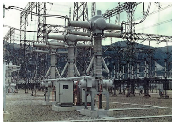
Fig. 8.35 A 240 kV double-pressure gas circuit breaker
