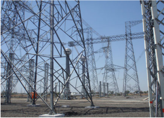
Fig. 11.43 1200 kV Bina National Test Substation, Madhya Pradesh (India), in 2013
