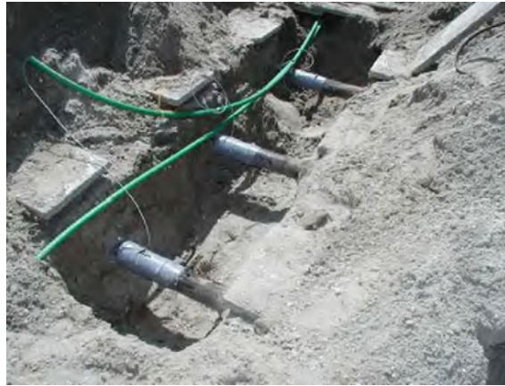
Fig. 10.50 150 kV cables with PT 100 elements at a hot-spot (adapted from [10.14])
