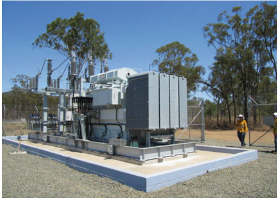
Fig. 11.41 Skid-mount substation example (Courtesy Ergon Energy, Queensland, Australia)
