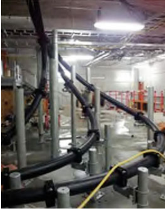
Fig. 10.106 Example of flexible constrained, snaked, and cleated cable installation arrangements (adapted from [10.14])
