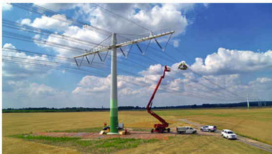
Fig. 9.178 Low-profile pylon of the CompactLine with composite V-strings—last works before commissioning in summer 2018 (source 50hertz)
