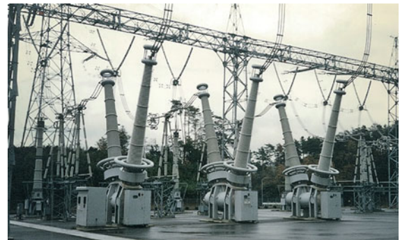
Fig. 8.5 Photograph of a 550 kV AC dead-tank circuit breaker. (Courtesy of Chugoku Electric Power)
