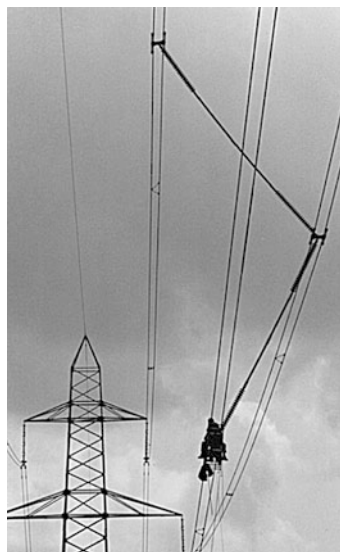
Fig. 9.100 400-kV interphase spacer in the transmission line at the Vorab Glacier in Switzerland (adapted from [9.194])
