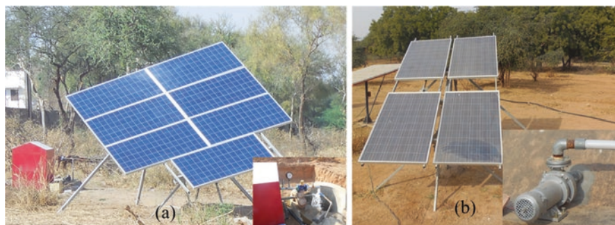
Fig. 11.1 Solar PV pumping system: (a) 1 HP AC pump and (b) 1 HP DC pump. (Source: CAZRI Annual Report 2013–14, pp. 89–90)
