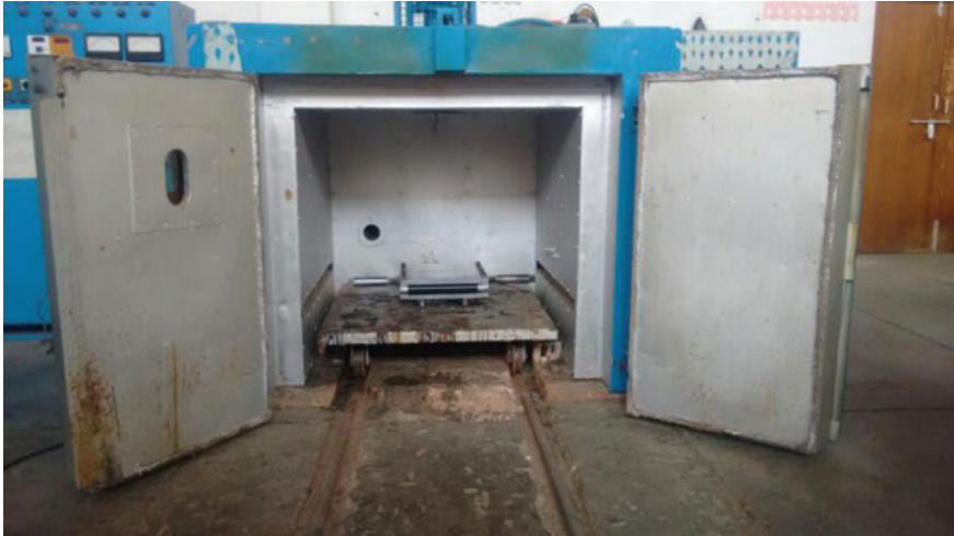
Fig. 65.2 Oven used for curing
