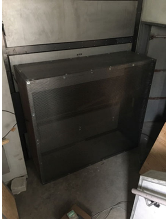
Photo 1 Dynamic pressure control system
