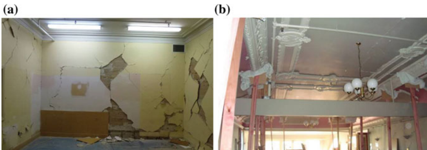
Fig. 2 Examples of the earthquake damages of McDougall House, including a the extensive cracking of the original lath and plaster wall system throughout the building, and b the cracking of the ornamental plasterwork ceiling within the Ballroom, with an exposed sprinkler pipework which detracts the value of this particular heritage fabric
