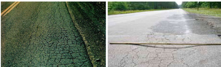
Fig. 1 Failures in pavements
