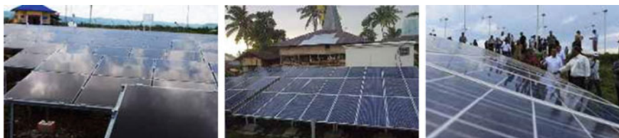
Fig. 19.7 Installed solar panel system
