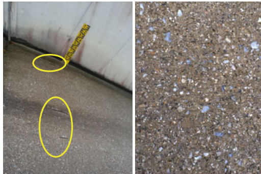
Lower part of the spillway – concrete is abraded and steel is visible
