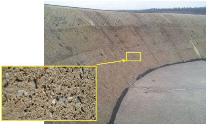
Weir – concrete is abraded
