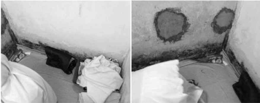
Fig. 15.5 (a) One of the unmaintained conditions of the prayer room. (b) The interior space in the prayer room in a shopping mall [4]
