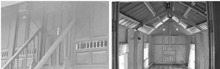
Fig. 23.7 Ventilation and lighting elements
