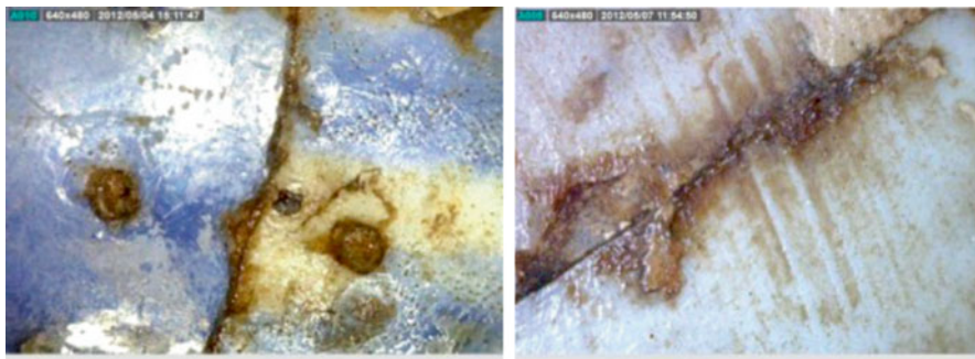
Fig. 13.3 Staining along the crack and inside the holes in the long term can cause permanent stain to the surface
