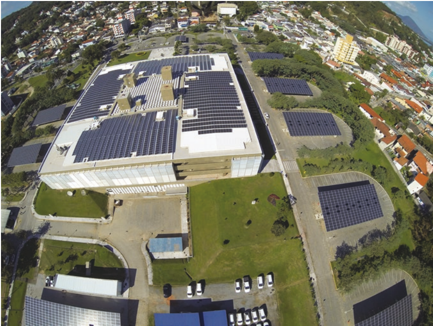
Fig. 7.11 Aerial view of the Eletrosul Megawatt Solar PV plant in Florianópolis, Brazil (27° South), showing the (450 kWp) rooftop and the nine parking canopies (565 kWp), which comprise the 1 MWp solar power plant
