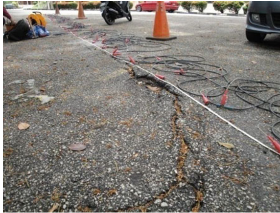
Fig. 3 Recording resistivity line at defect of transverse cracking
