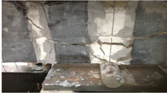
Fig. 4 Cracking and failure pattern of beam C2.5-UA-V1
