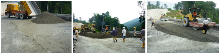
Fig. 6 RCC transporting, spreading, and compacting, nuclear density meter used to check the density every layer of RCC placement completed
