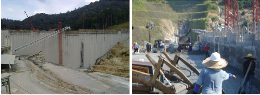
Fig. 5 Conveyor system apply at Batu Hampar dam when the RCC level reach higher level
