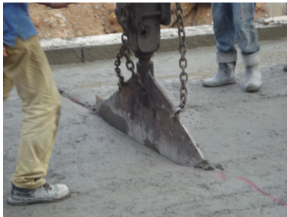
Fig. 7 Transverse joint were cut and installed a galvanize thin plate at Batu Hampar dam
