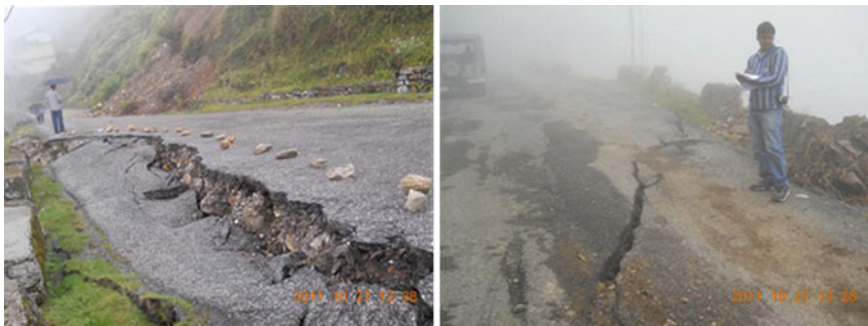
Fig. 1.4 Cracks and subsidence, Nathula-Gangtok Road, Sikkim-Darjiling Himalaya (Source GSI, Engineering Division, Gangtok, Sikkim)
