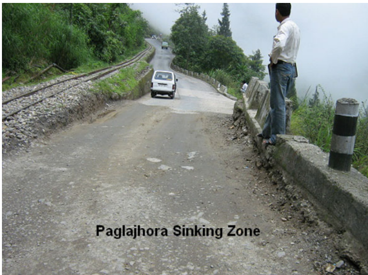
Fig. 8.19 Road subsidence at Paglajhora
