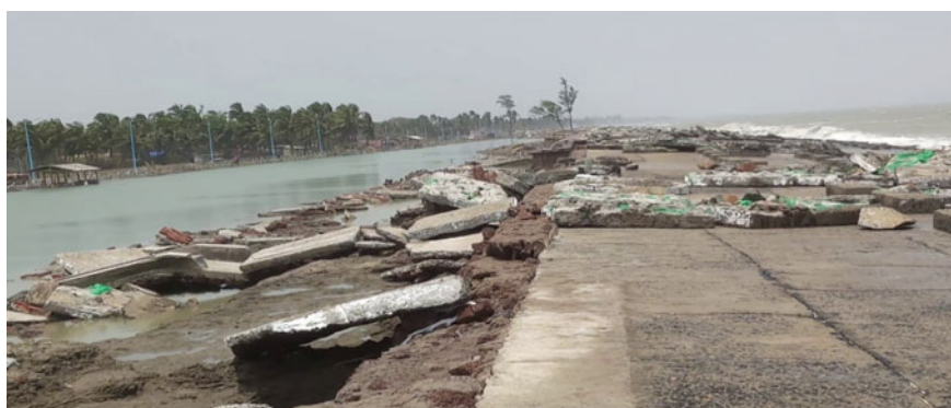
Fig. 3 Damaged sea wall in country side at Shankarpur bus stand as observed on 28.5.2021
