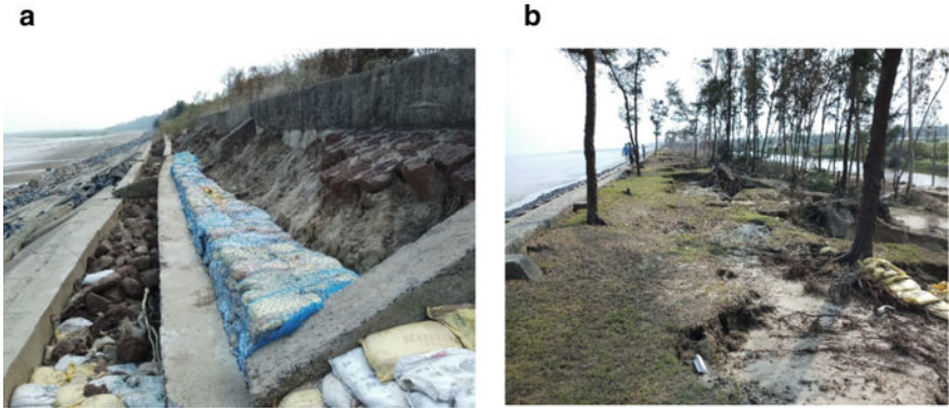
Fig. 10 a and b Damaged Sea Wall at Bankiput, near Junput as observed on 29.5.2021
