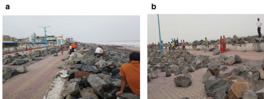
Fig. 8 a Stone boulders from sea face slope, got accumulated near and b Guard wall overtopped to C/S as observed on 28.5.2021
