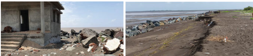
Fig. 2 Erosion at Nani Danti Moti Danti Site
