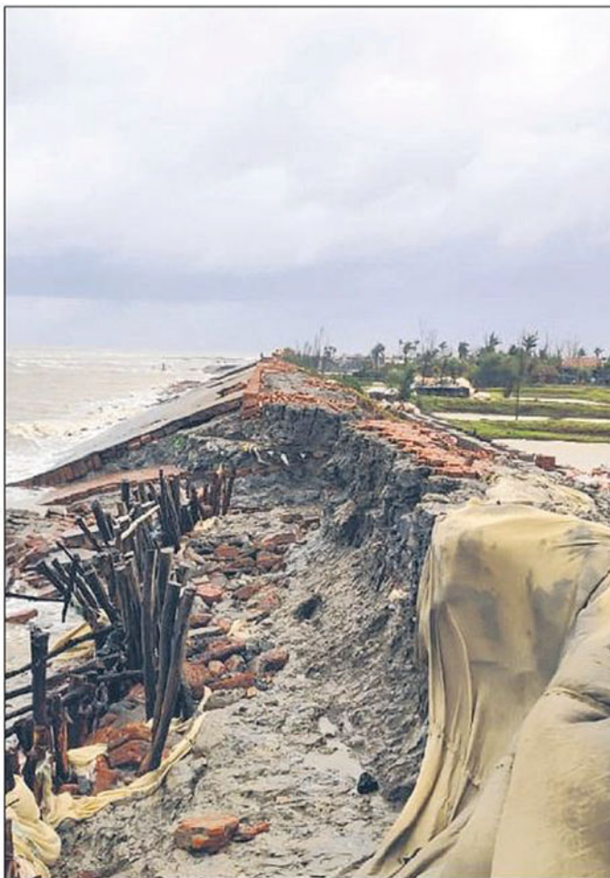
Fig. 14 Embankment breach in G-Plot area of South 24 Parganas as observed on 26.5.2021
